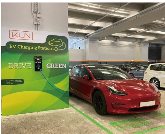
Four EV charging stations were installed at Kerry Cargo Centre in Hong Kong in the fourth quarter of 2021 to allow employees to conveniently charge their cars and to encourage the use of EV
